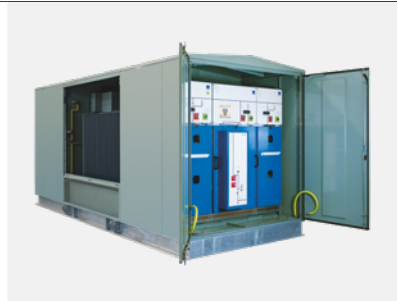
Medium Voltage Equipment
